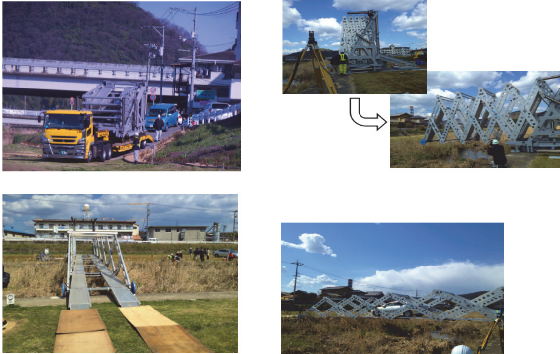
Fig. 4 Experimental conditions of erection on a real river: bridge transport (upper left), Erection status elongation status (upper right), after construction (lower left) and vehicle driving tests (lower right) [4].
